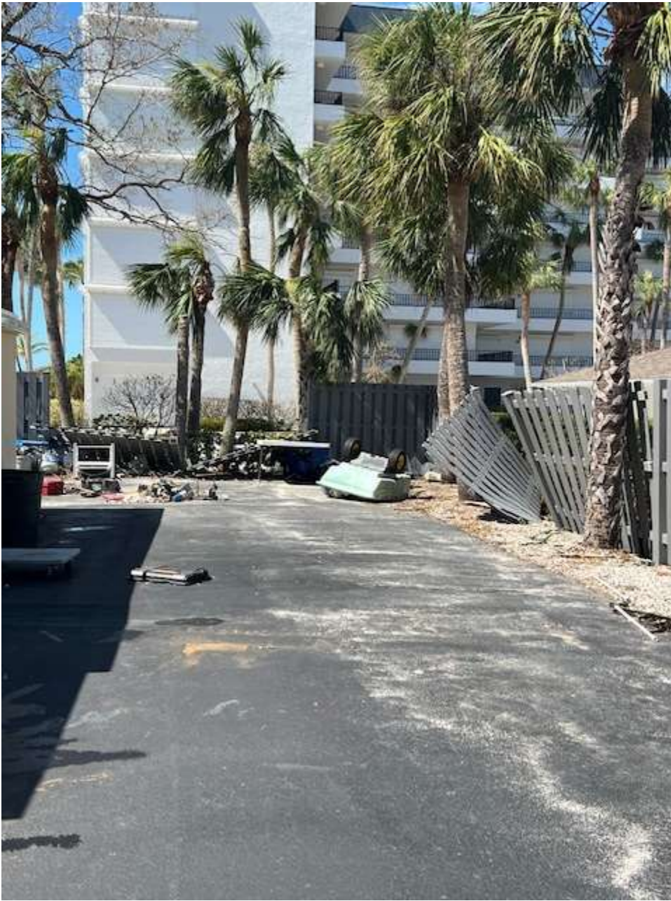
Maintenance area fence damage
